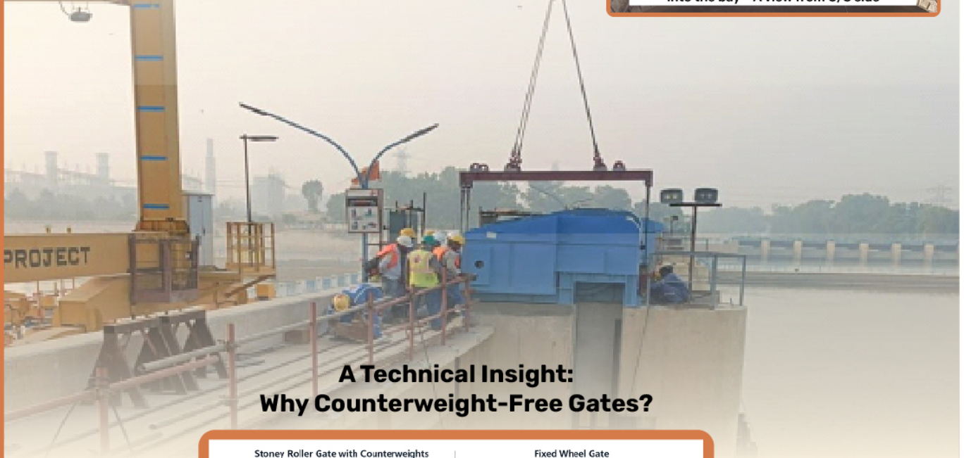
Sukkur: Lowering down of the Gate-section into the bay - A view from U/S side
