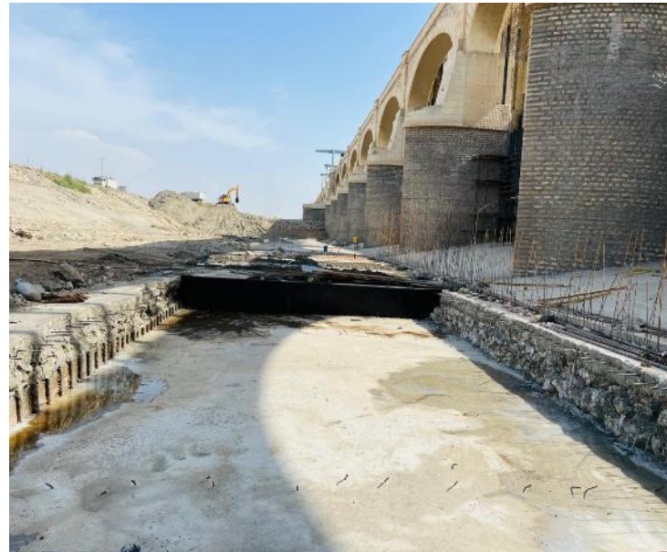
Settled U/S apron at bays 15 to 17
