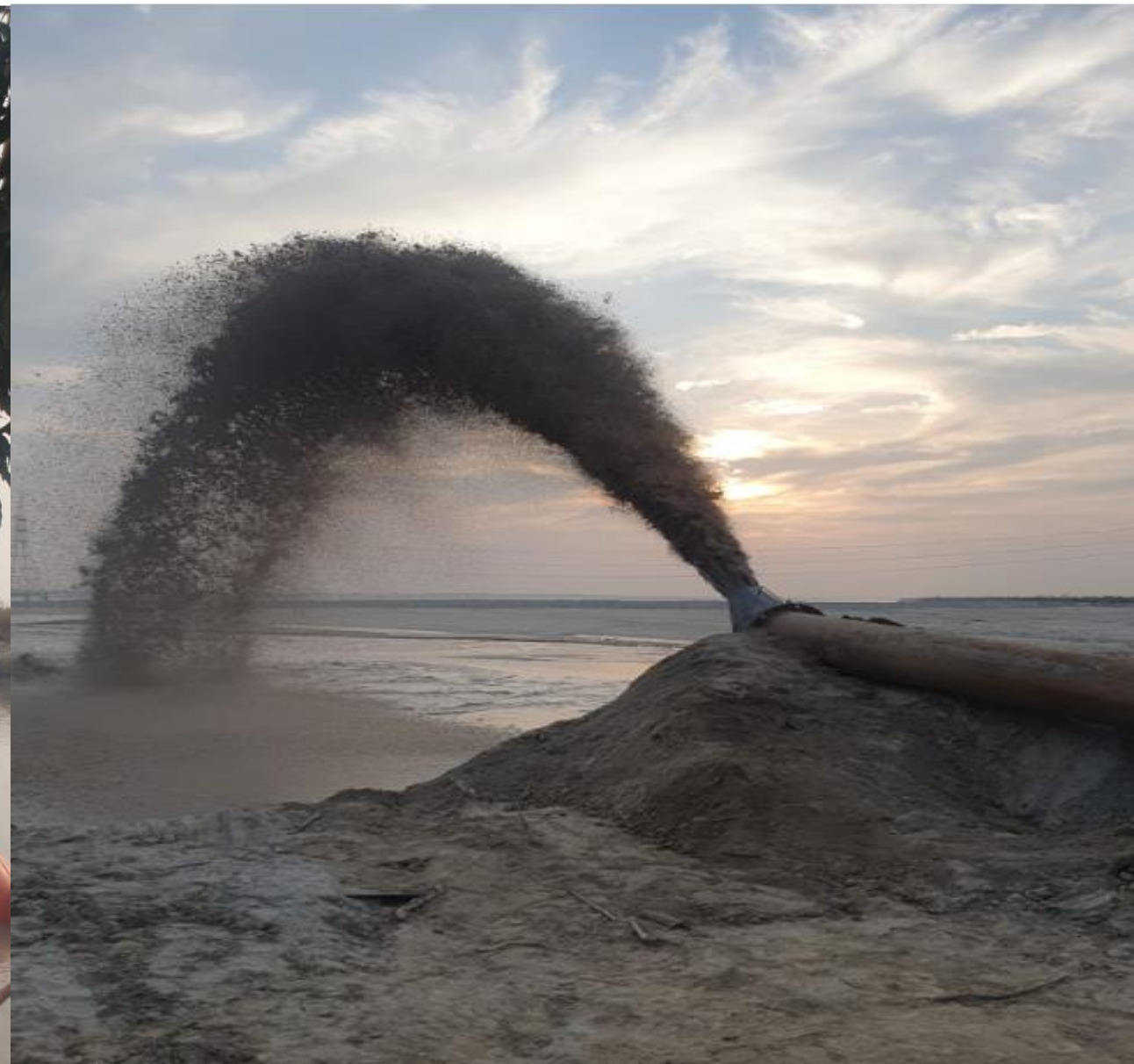
S1 – Disposal pipeline in containment bund
